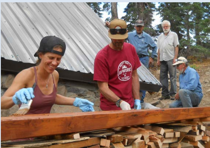
Bethany Hinchliffe (left) and Chris Edmands (center) staining 4x4 rafter supports at Benson.
