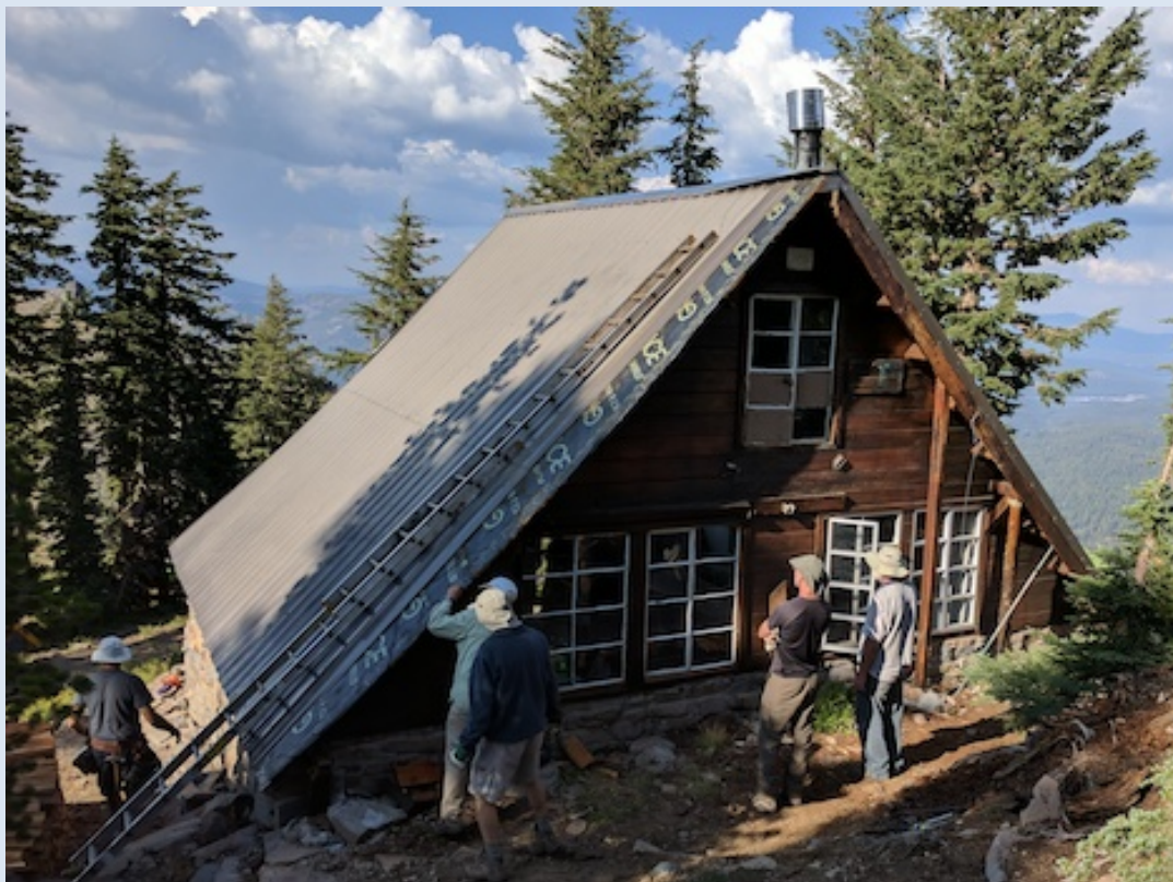
South side of Benson Hut after barge rafter demolition (photo by Peter Race).
