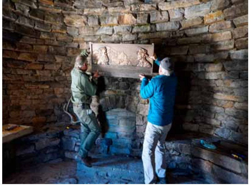
NPS's Thor Riksheim and Doug Harnsberger install the new Muir Shelter plaque
